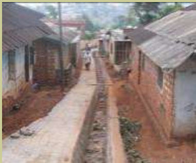
Improved water drainage thanks to LED
